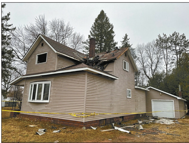
A home on North State St. sustained fire damage after a middle-of-the-night fire during a lightning storm April 12/13, 2022.
