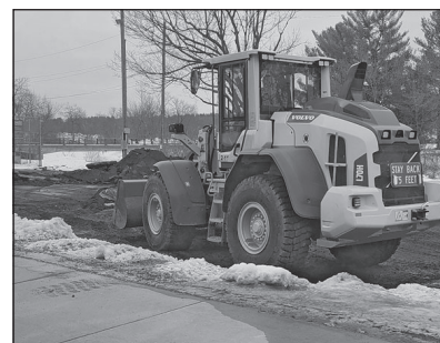
The tennis courts across from the T.B. Scott Library being removed in early March. MMC Staff photo.
