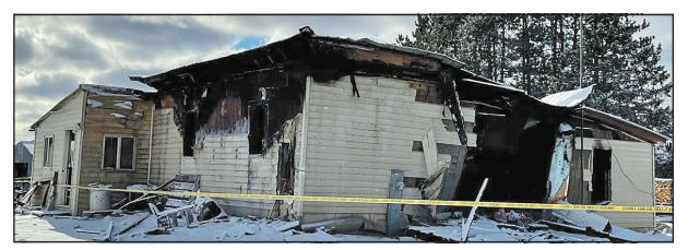
This home in the Town of Pine River is a total loss as the result of an early morning fire last Friday, Dec. 17, which also took the life of one occupant of the home. Tina L. Scott photo.
