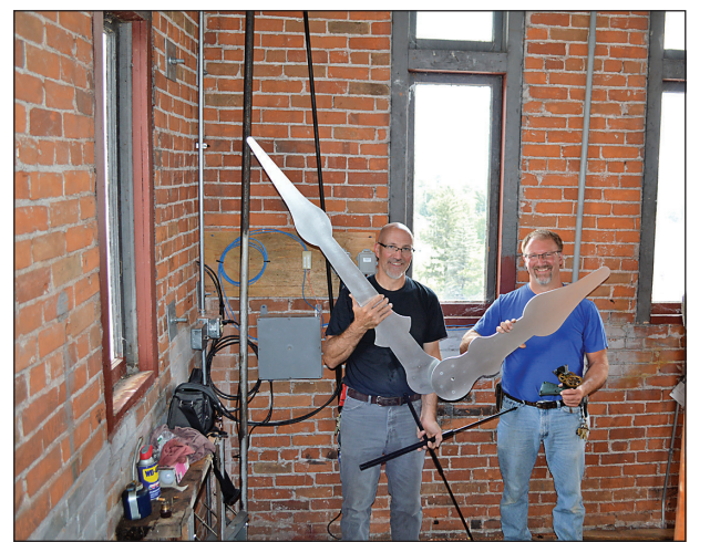
Pat Gierl (left) and Andy Rudolph prepare to ascend to the clock tower with the new hands and gear box. Michael J. Caylor, Jr. photo.
