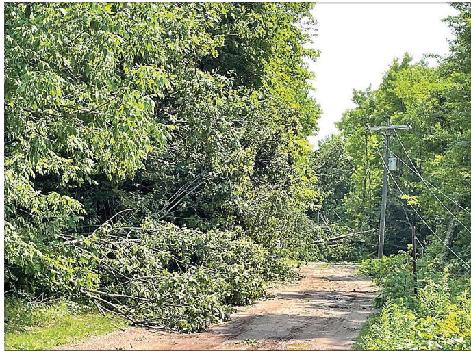
Downed power lines throughout the area caused widespread power outages as a result of Monday and Wednesday evening storms. Here trees and downed power lines block a driveway off of Hwy. K north of Merrill.
