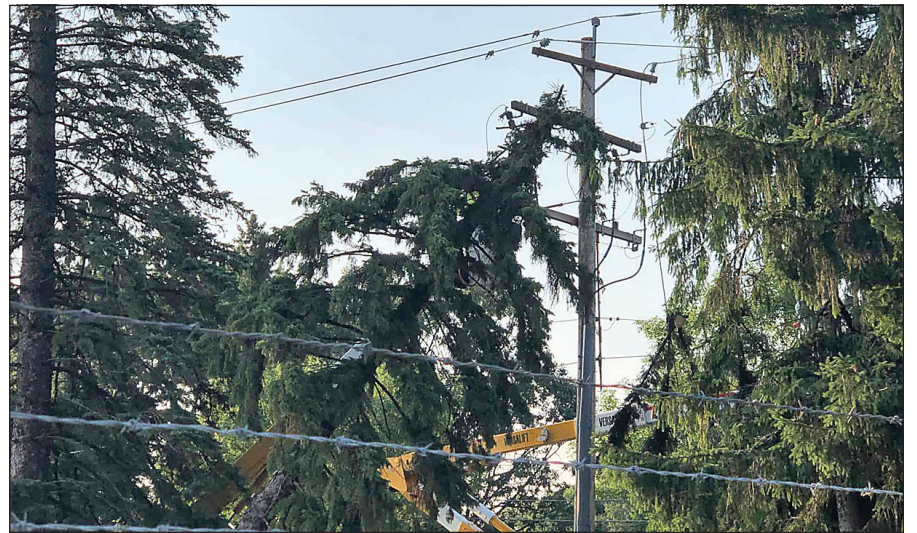
Trees and power lines were damaged throughout the area.
